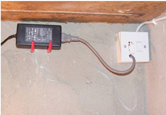
Figure 11-11. The 12V DC power supply
