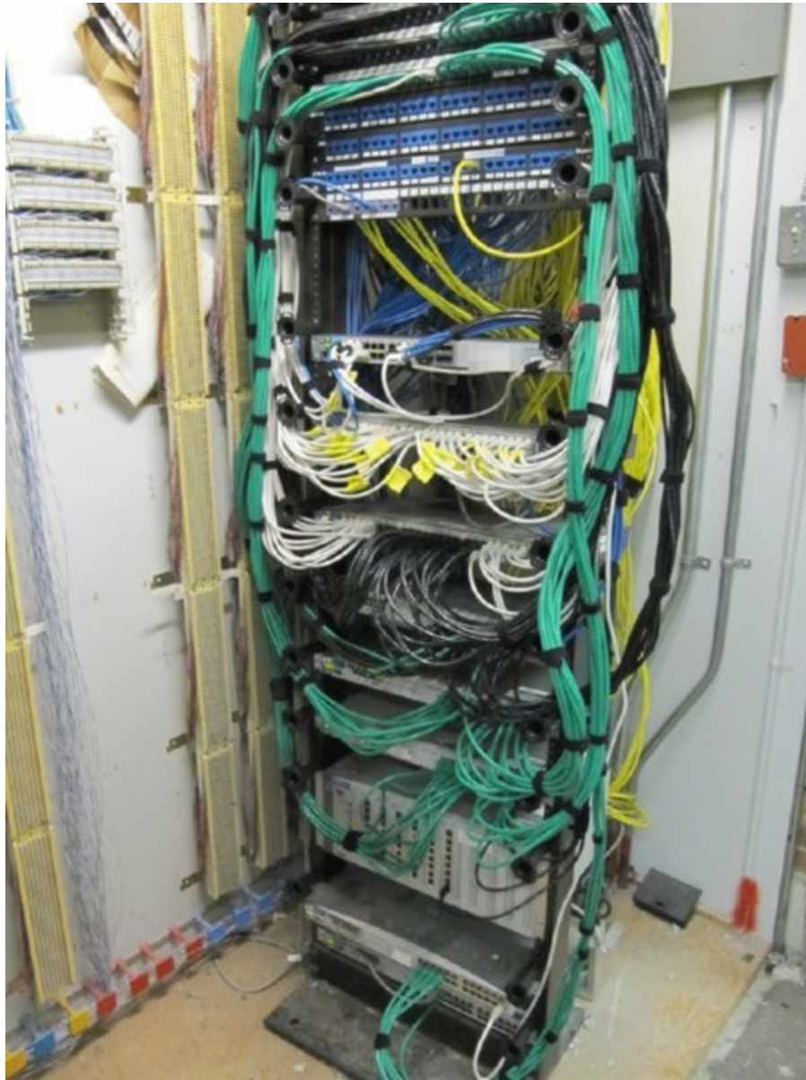
Figure 10.1 A typical wiring closet
