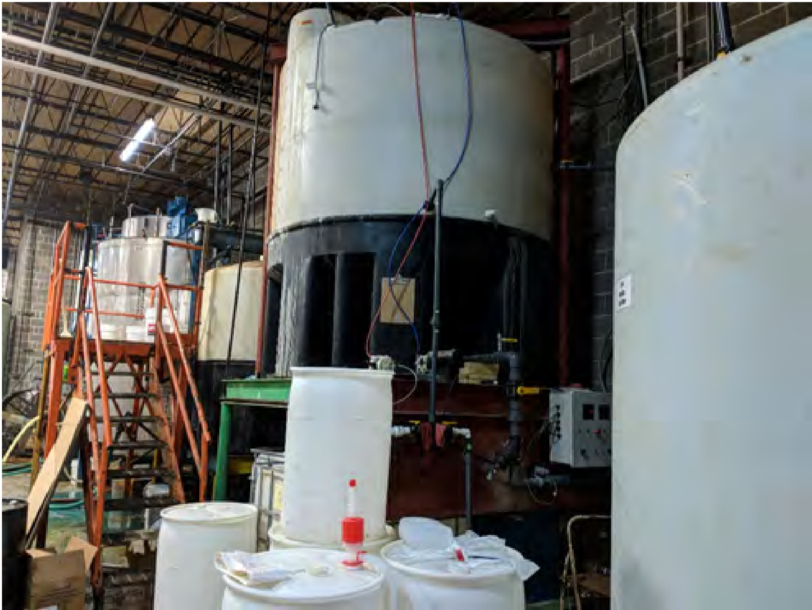
Figure 8H: Acid and caustic tanks: These tanks hold the acid and caustic needed to balance the PH of the wastewater produced from a large agriculture components metal coating process.
