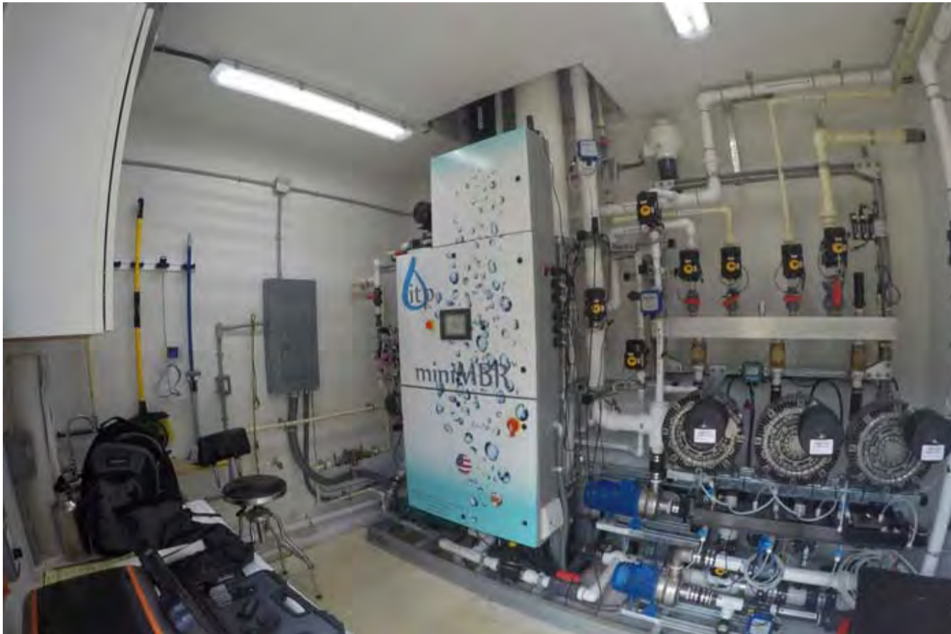
Figure 8L: Multiple control panels and valves. Whether it's the largest or smallest MBR-equipped plant, the equipment and control strategy are very similar. A typical unit uses 14 automated valves, four pumps and three blowers. (Source: ITP)
